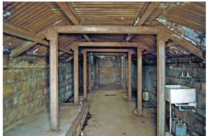
Many of Nottingham's pubs had medieval and later rock-cut cellars (one described as a cock-pit!) which were ideal for use as shelters for the owners and customers with a little adaptation
